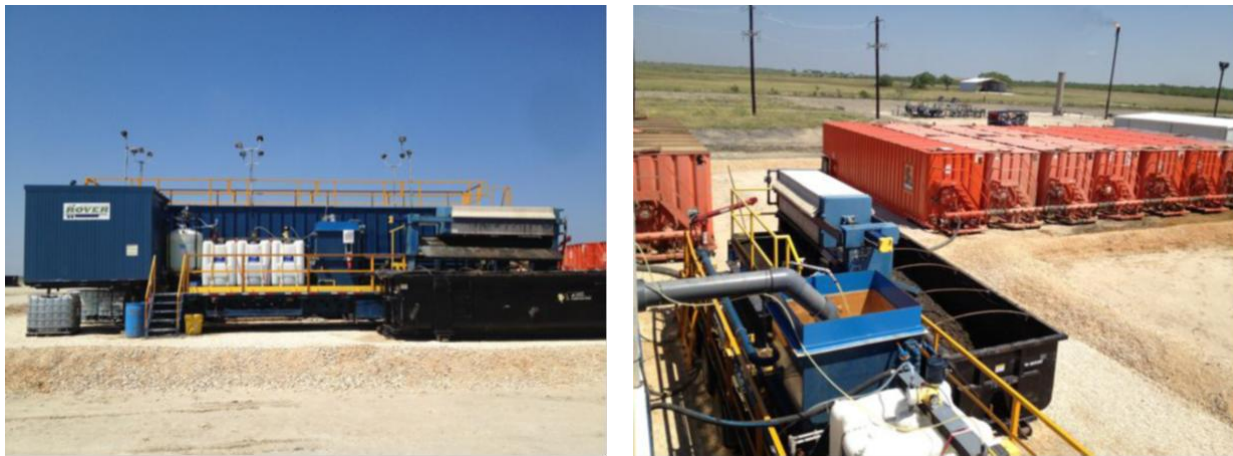
Figure 8: Photographs of the ROVER Re-Use Facility (Left and Right)
